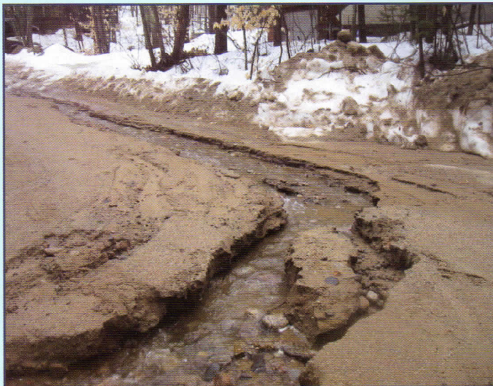
Photo 1: Runoff water caused this rural road to be eroded away.
