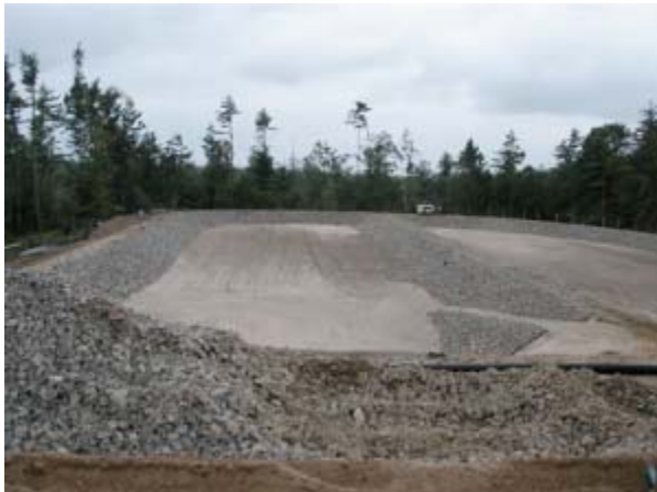
The nearly completed Rapid Infiltration Basin for Wolfeboro's sewage treatment project. (Courtesy David Ford)
